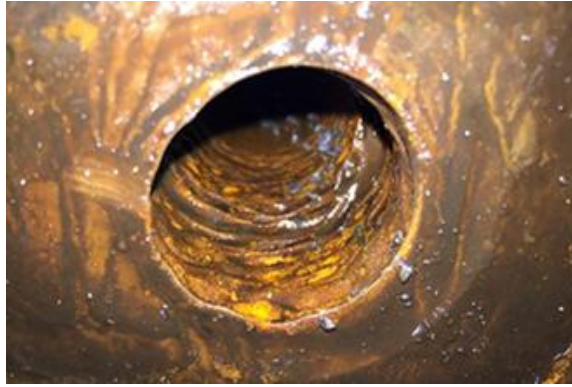
Fig 4. Erosion Caused by Sand in the Valve [11]
